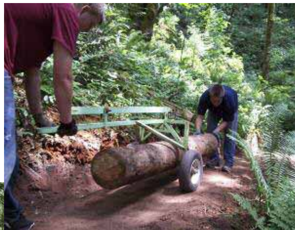
Two of the Community Solutions summer crew use a junior arch to move a large treated pole into place for a stream crossing on Little Buckner Trail.
