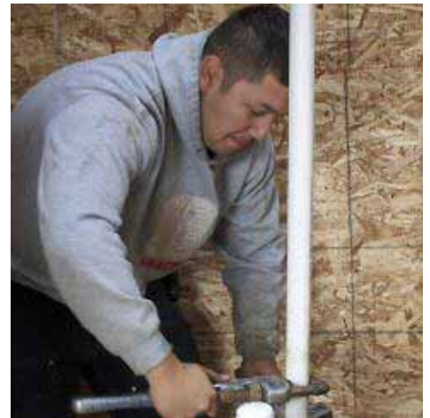
While some construction activities are on hold at this time, recently a crew from Fisher's Supply in Canby, Oregon inserted the pump and waterline into the well that was drilled in May 2008.
